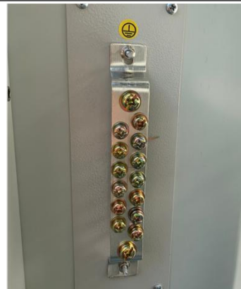
Cooper grounding bar
